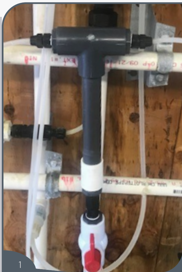
An in-line chamber provides improved reaction time for chlorine dioxide.
