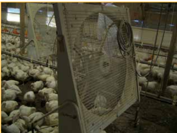
Figure 100: Circulation fans in a naturally ventilated house.
