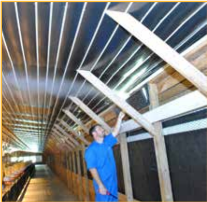
Figure 106: Using a smoke test to determine if air flow and operating pressure is correct.
