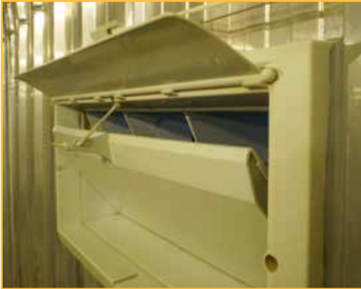
Figure 109: Example of a good-quality air inlet.
