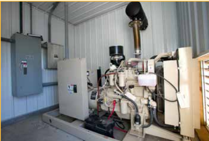
Figure 97: Example of a back-up generator.
