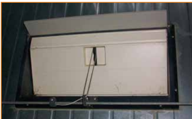
Figure 6.9: Example of a good-quality air inlet.
