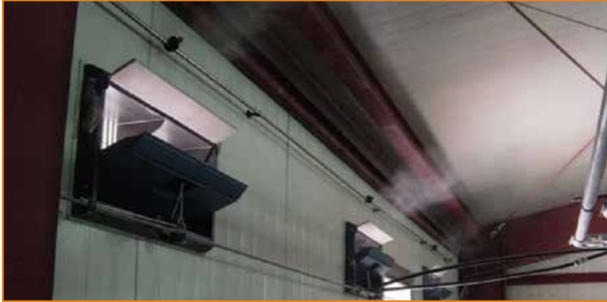
Figure 6.21: Example fogging system for a cross-ventilated house.
