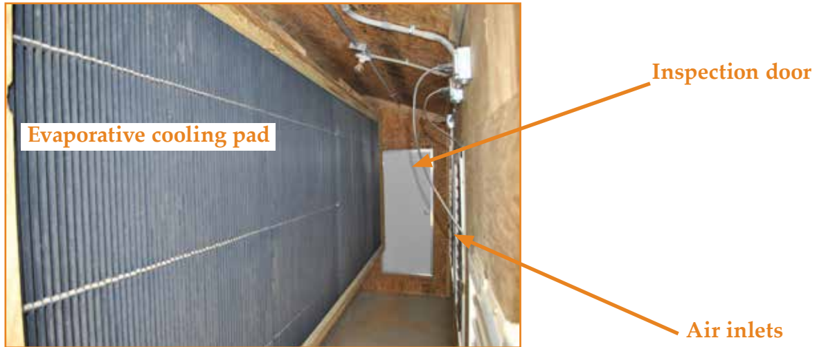
Figure 6.20: Example of a cooling pad installed on the sidewall of the house in a doghouse.
