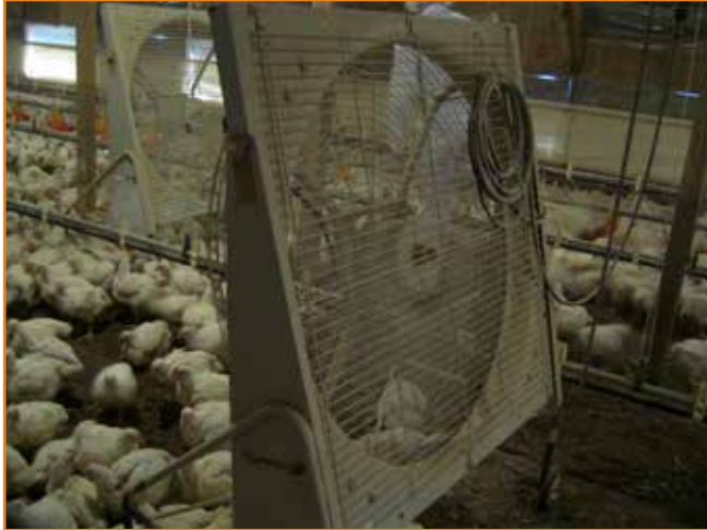
Figure 6.2: Circulation fans in a naturally ventilated house.
