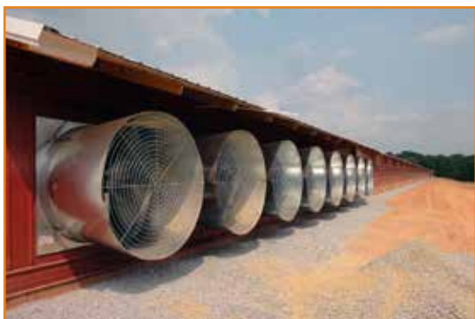
Figure 6.13: Example of a typical tunnel ventilated house.
