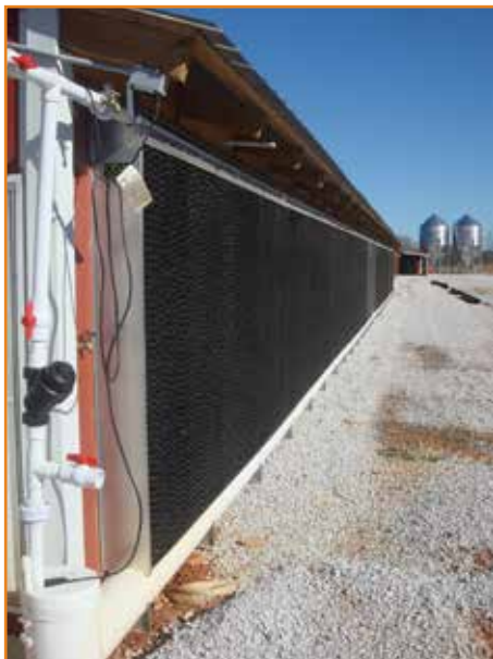
Figure 6.19: Pad cooling with tunnel ventilation.
