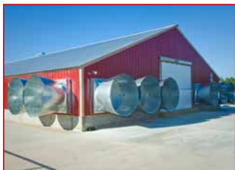
Figure 112: Example of a typical tunnel-ventilated house.
