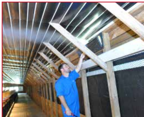
Figure 106: Using a smoke test to determine if air flow and operating pressure is correct.
