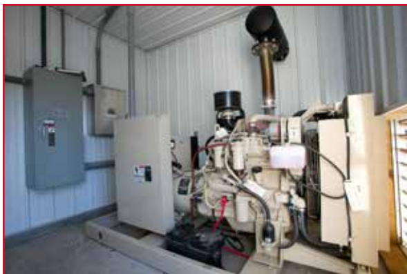
Figure 97: Example of a back-up generator.
