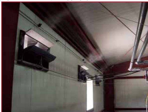
Figure 118: Example fogging system for a cross-ventilated house.
