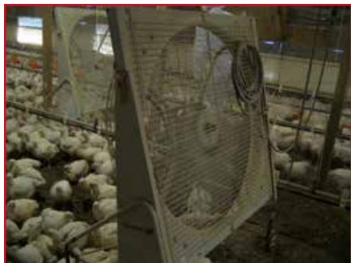
Figure 100: Circulation fans in a naturally ventilated house.
